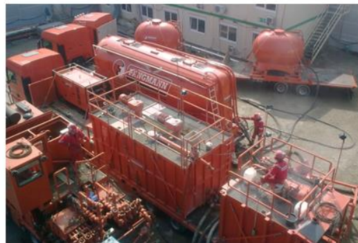
Figure 5: Pumping profile and equipment on site
